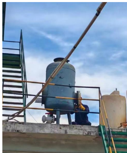
活性炭吸附罐
