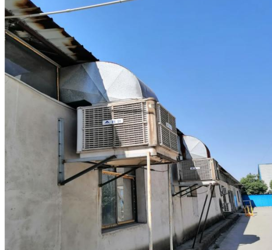
丝印车间废气净化设施
